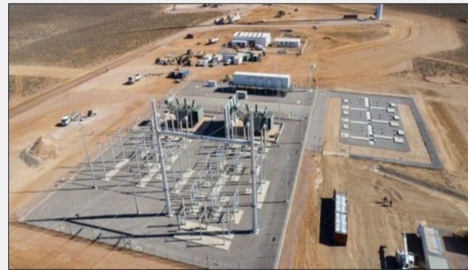
Collector substation – including 33/330kV power transformers
