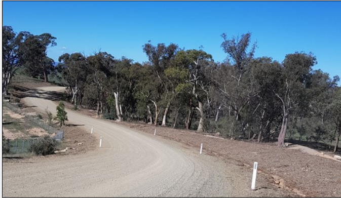
Access tracks – 5 to 6m trafficable width; plus cut / fill batters; drainage and erosion control; cable trenches
